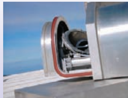
Photo 5. FTIR Solar tracker on the roof of the new container
